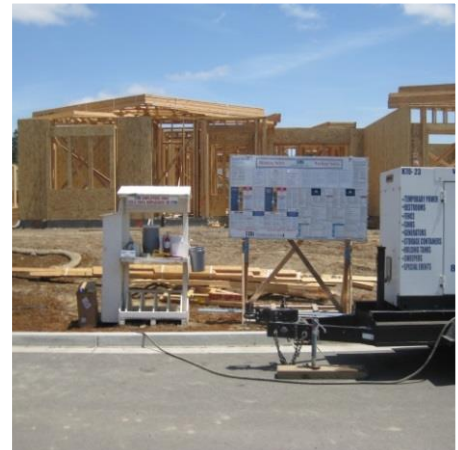
Safety Station and Postings
